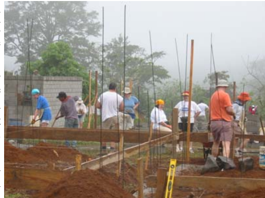
Members of the Habitat build team work through some damp weather while working on three houses.
